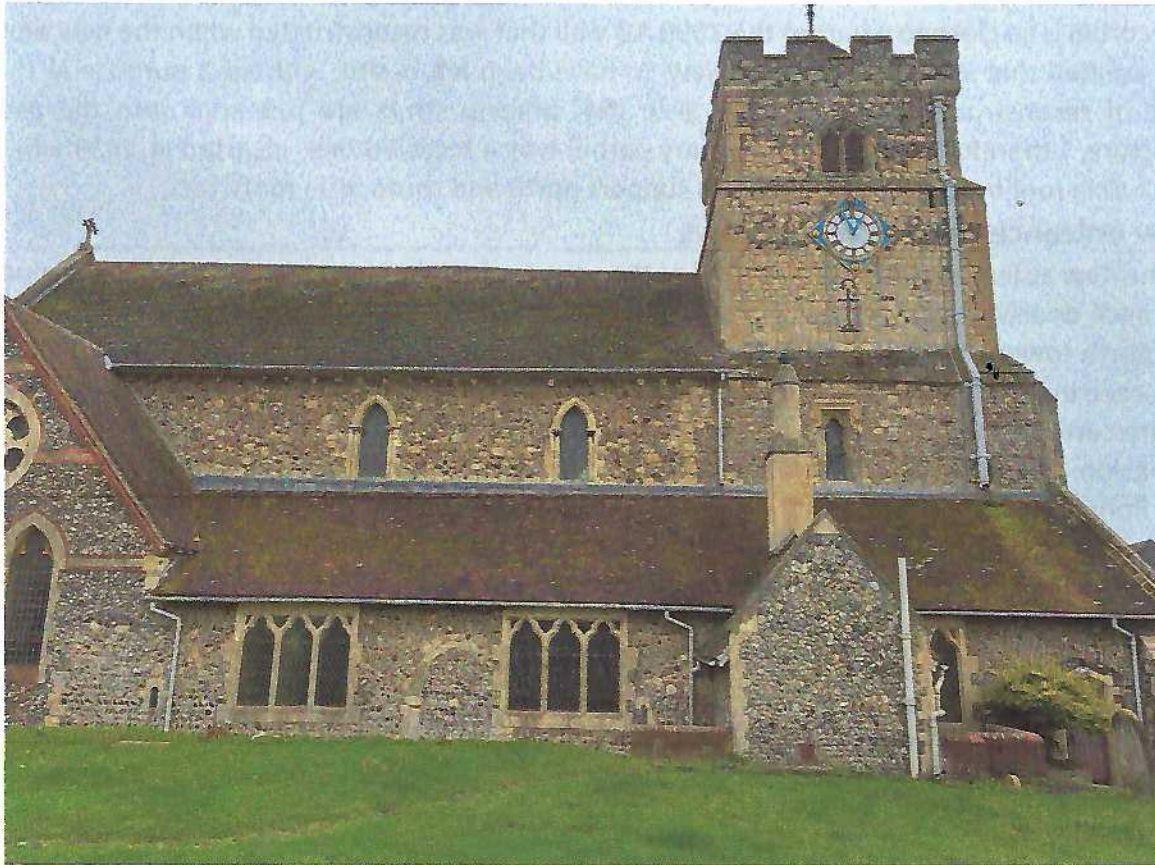
Fig 9a North façade of the church with 1200 doorway and slit windows (2 in view)
