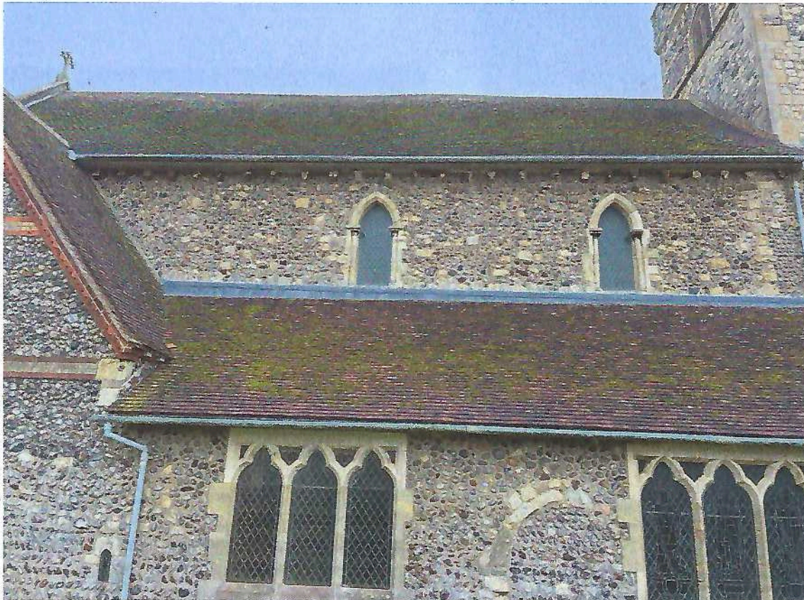
Fig 9b 26 new and old corbels along the north clerestory wall plate
